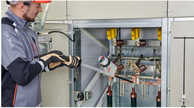
PHE4 voltage detector with visual and acoustic indication.
