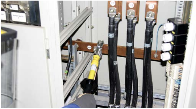
Attaching an earthing and short-circuiting device in a low-voltage switchgear installation using an earthing handle.
