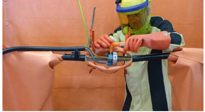
Covering live parts.
