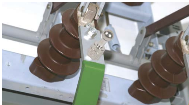
Straight fixed ball point mounted on a busbar.
