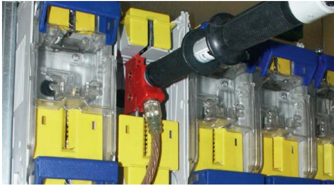
Attaching a fully insulated earthing and short-circuiting device using an earthing handle of type VI.
