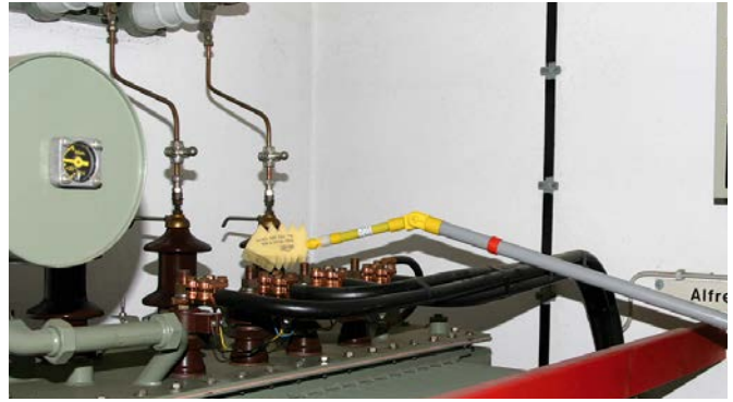
Damp cleaning of a transformer using the FRS ZK MS damp cleaning kit.
