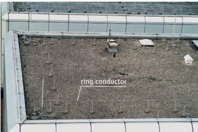
Fig. 9: Roof-mounted air-termination rod and elevated ring conductor with connection to the isolated down conductor
