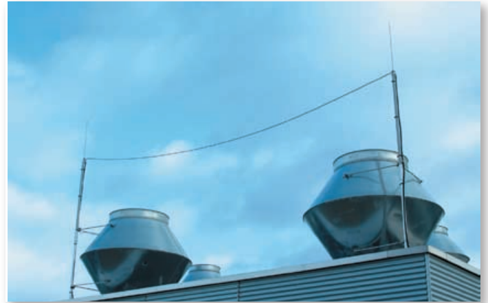
Fig. 8: Roof-mounted ventilation system with electrically isolated air termination system and spanned cables
