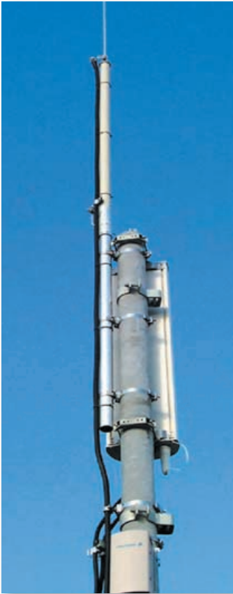
Fig. 7: The DEHNconductor system with the HVI isolated down conductor used to provide electrical isolation of a 2G/3G antenna system from the building
